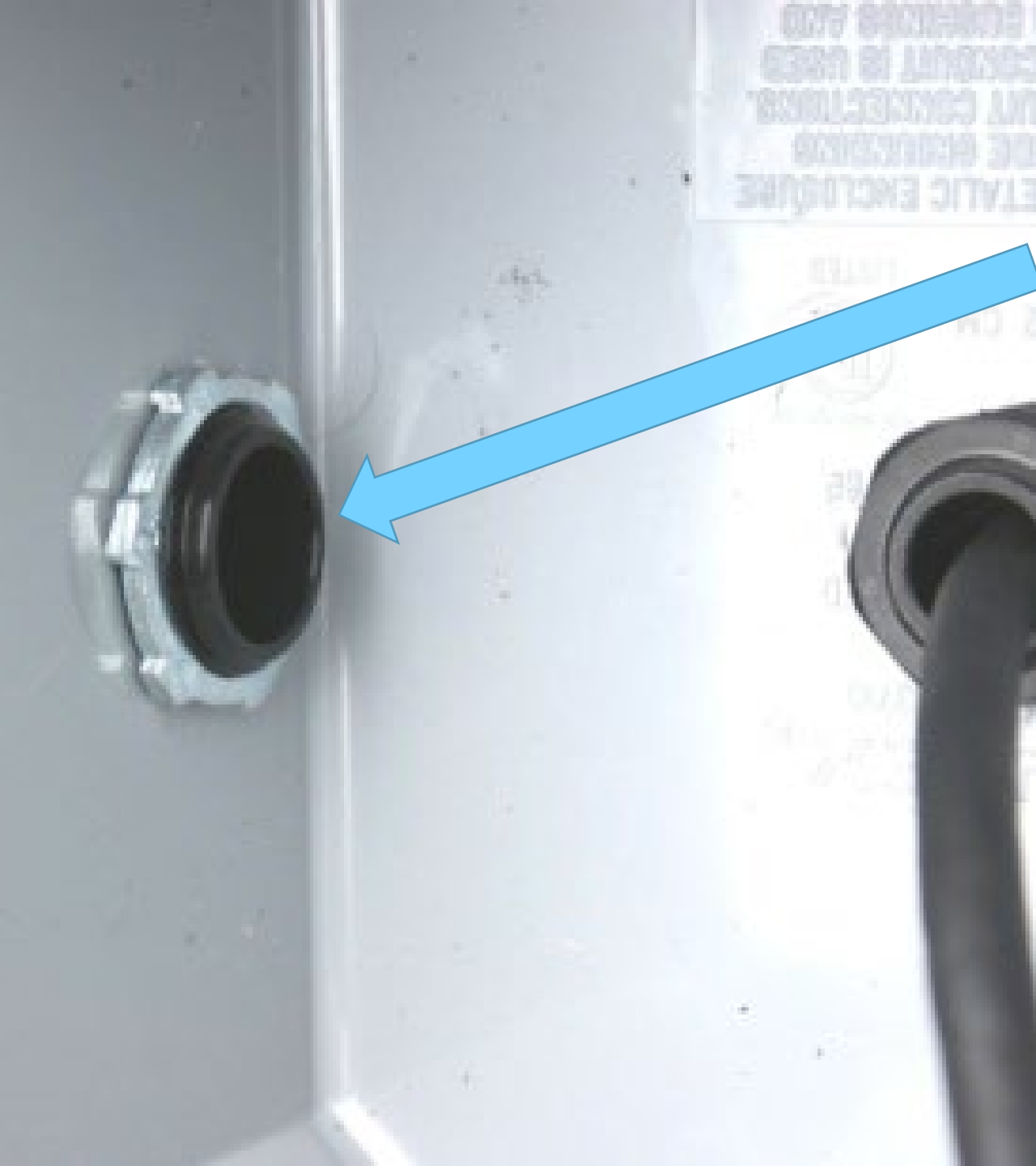
Watertight Conduit Connector Nut Inside of the Junction Box
